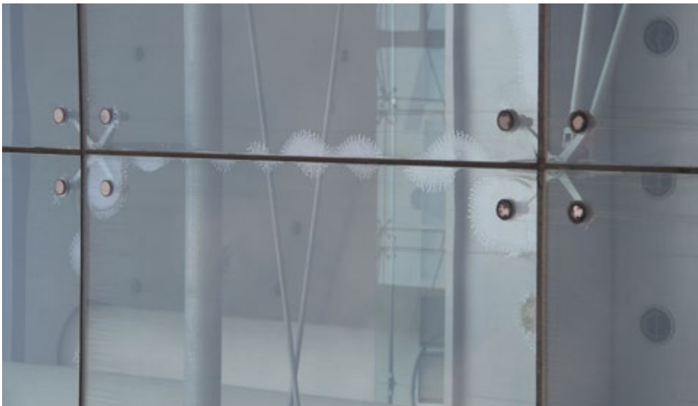
Typical defects caused by delamination.
